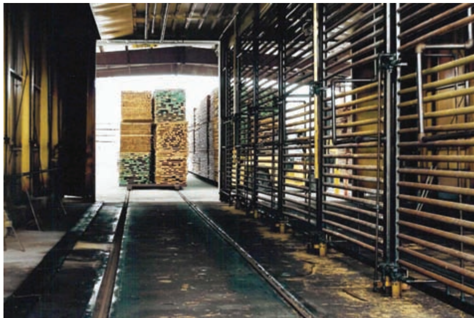
View of a full tram load of lumber from inside of double track American Wood Dryer kiln.
